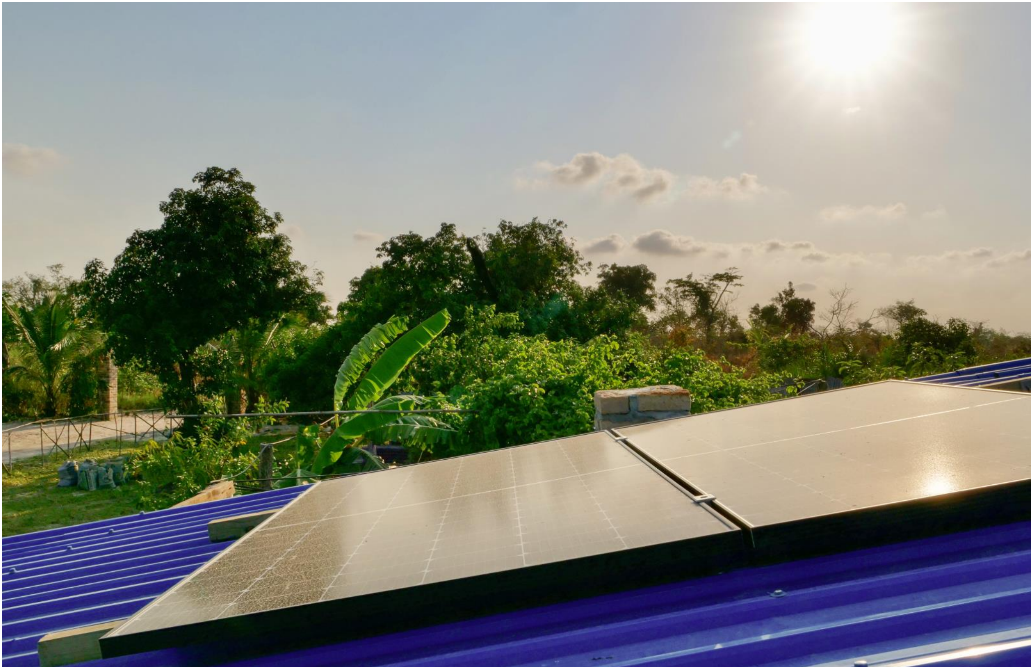
The sun, God's gift to make electrical power where there is no chance of getting access to the grid.
