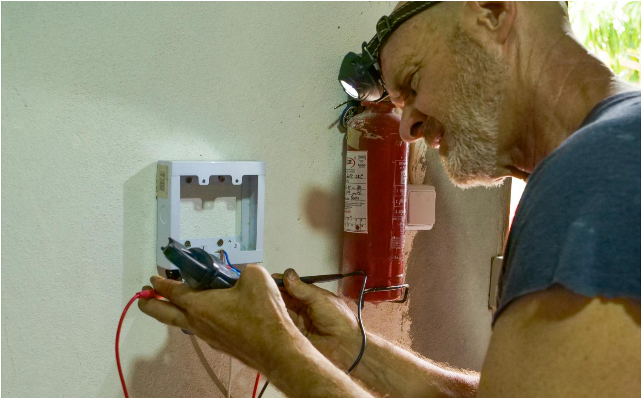
Mercy Air volunteer, Bruce, is a solar expert. He arranged everything, from sourcing the equipment to completely installing the solar system.
